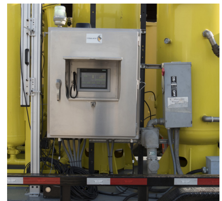
Control panel for monitoring air pressure, temperature and more.
